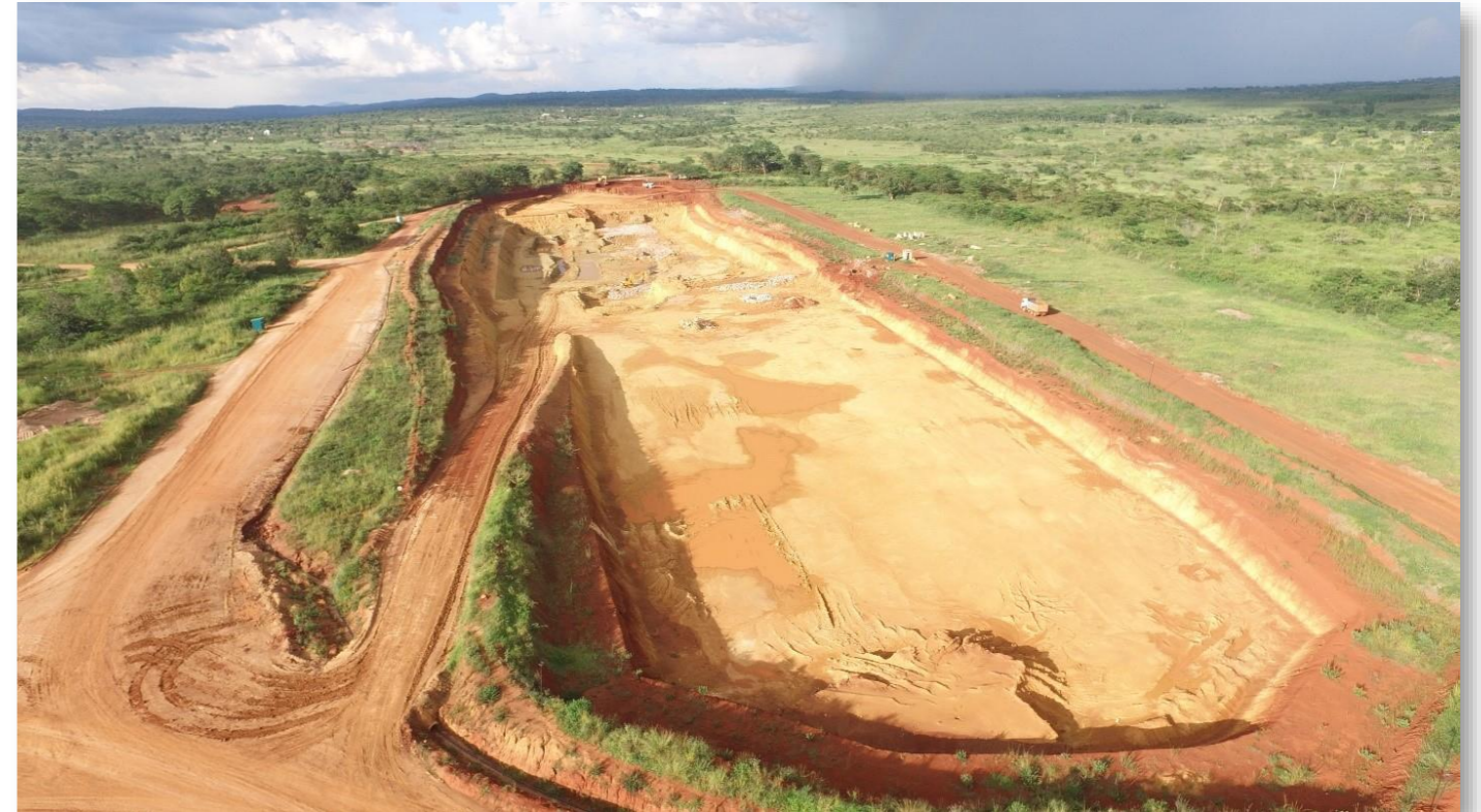
BUCKREEF GOLD OPEN PIT (MAY 2022) WITH VIEW TOWARDS NORTH-EAST AND DRILL RIG LOCATION
