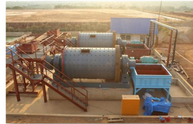
Ball mills installed
