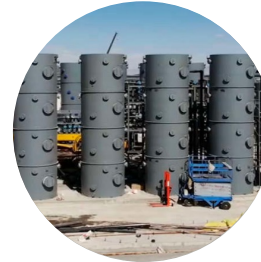
Existing DLE plant
