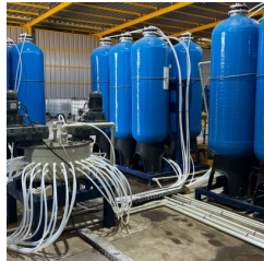
CTL's DLE Pilot Plant in Copiapó
