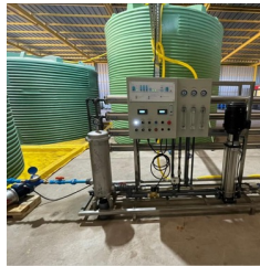
CTL's Reverse Osmosis Unit in Copiapó
